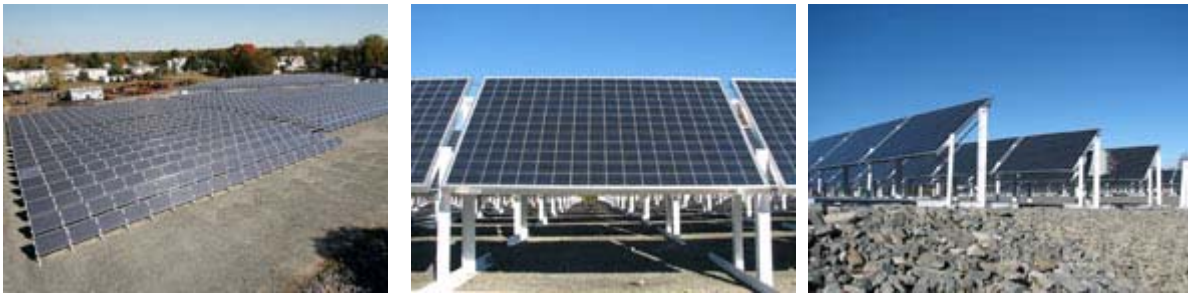
Figure 1. These images depict the Brightfield solar power plant in Brockton, Massachusetts. Source: Waste News; 29NOV08.
